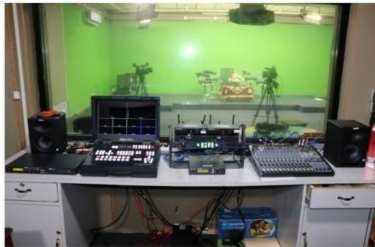
PRODUCTION CONTROL ROOM (PCR) EQUIPPED WITH HS 1300 DATA VIDEO SWITCHER
